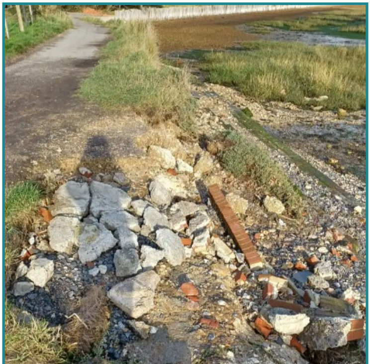
Damaged seawall © Coastal Partners
